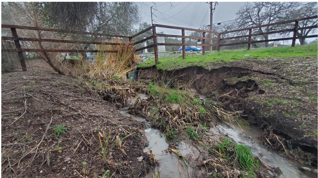
Stream bank erosion worsened January 2023
