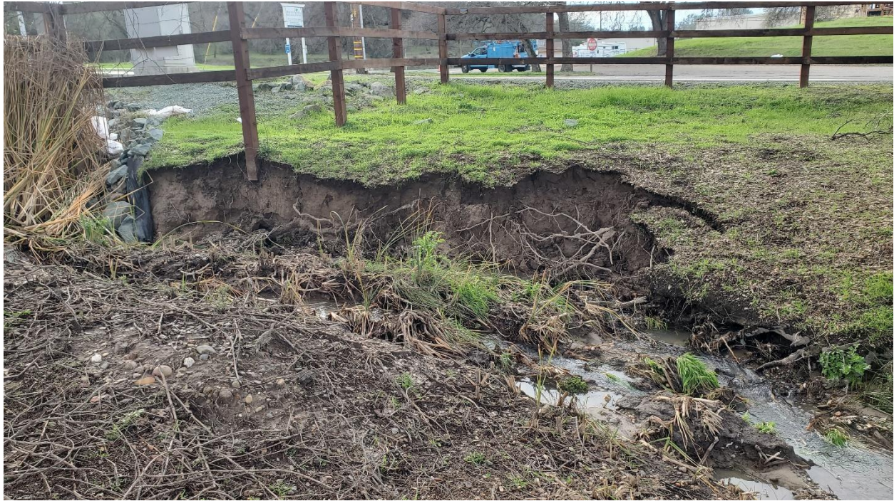
March 2023 erosion exposes a fencepost and a fracture forms threatening an oak tree just downstream
