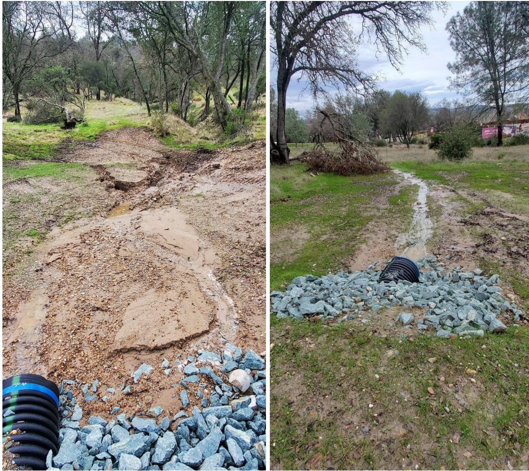
Eroding tributary from BV Peak property that feeds into the western stream during storm events. This is a candidate for stormwater control bioswale project. Photographed January 2023
